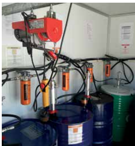
Storage area for bulk lubricants
