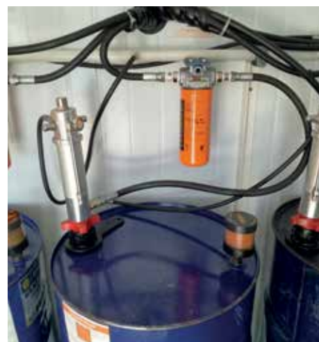
Storage area for bulk lubricants
