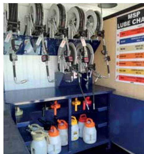
Dispensing bay area inside the lubrication container
