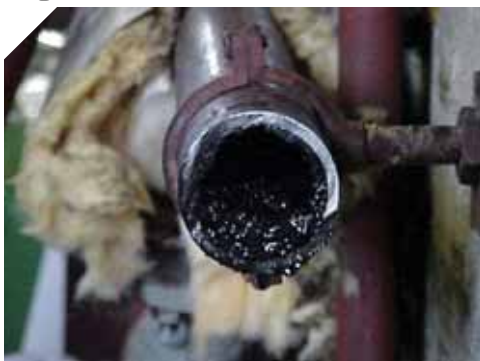
The new heat transfer oil test promotes industrial efficiency by preventing your system from failure such as this.
